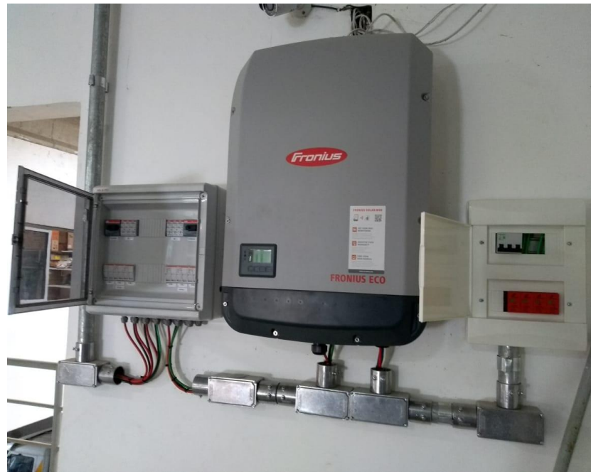
Figura 23-String box CC - Inversor- String box CA
