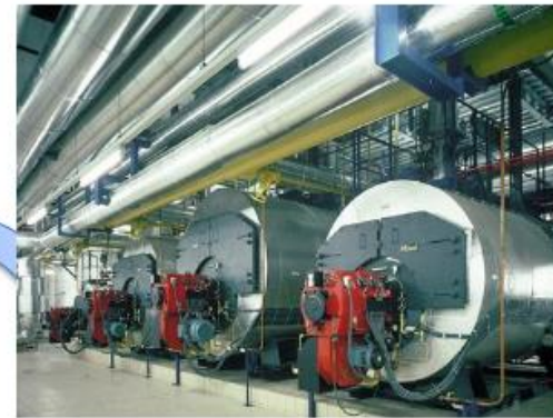
Industrial process heat
