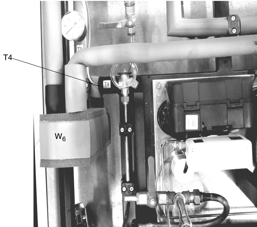
Fig. 3.2 Top view of one part of the refrigeration set
